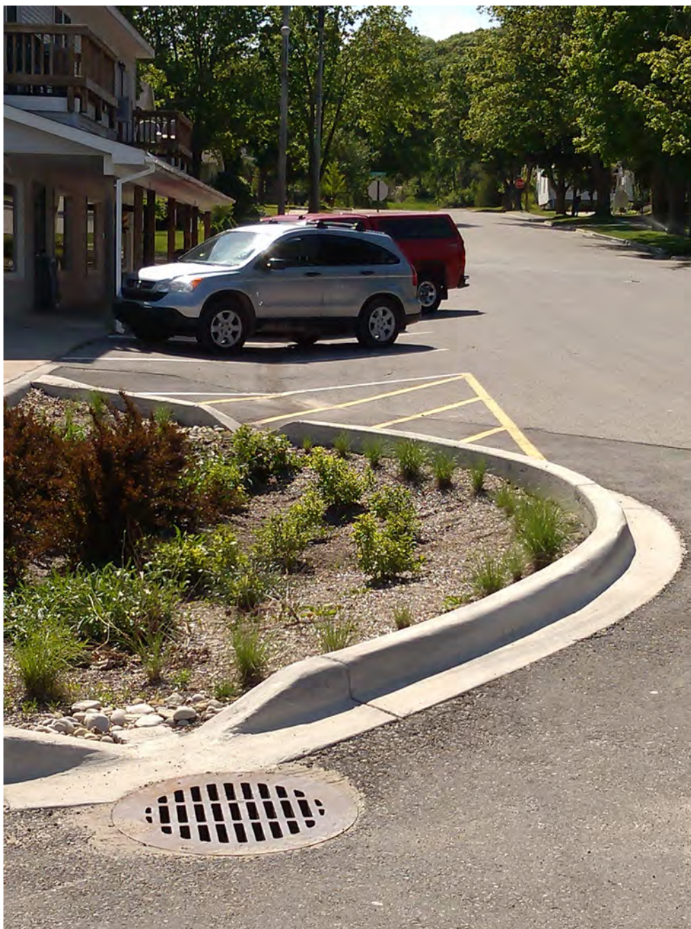
Planning for stormwater management can include controlling the amount, quality, and timing of runoff to prevent its damaging effects on natural resources. Curb cut-outs allow stormwater to flow into this garden and soak into the ground. This helps clean the water before soaking into the ground. The storm sewer allows for overflows to prevent flooding. Photo: DEQ
